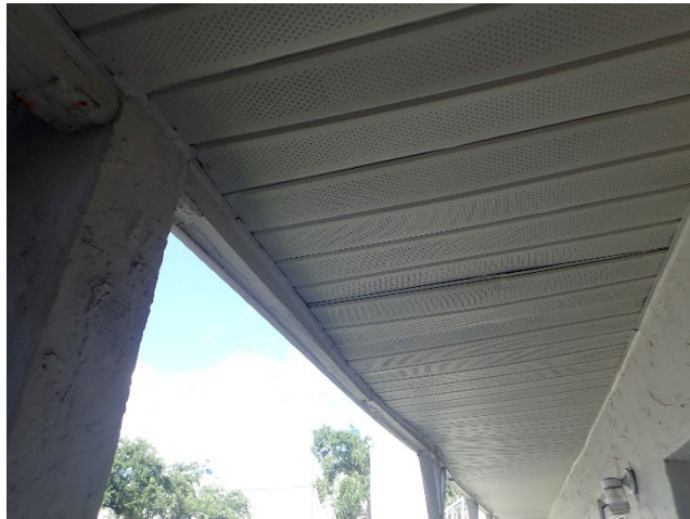
Distorted aluminum soffit at Building 4
