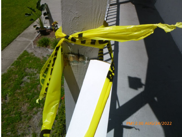
Broken handrail connection at Building 13
