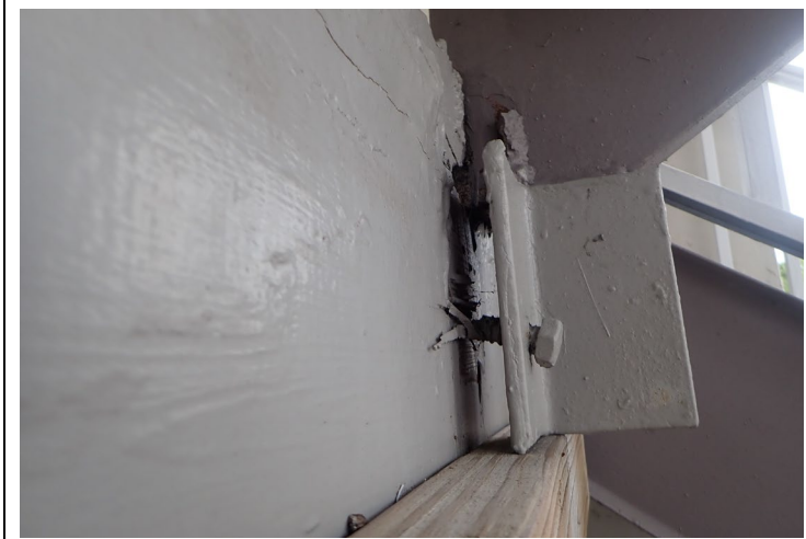
Loose screw at metal stairs of Building 11
