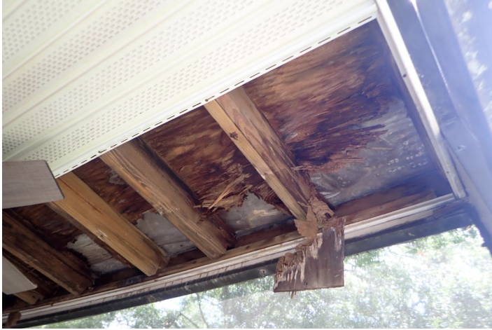
Deteriorated framing at Building 22
