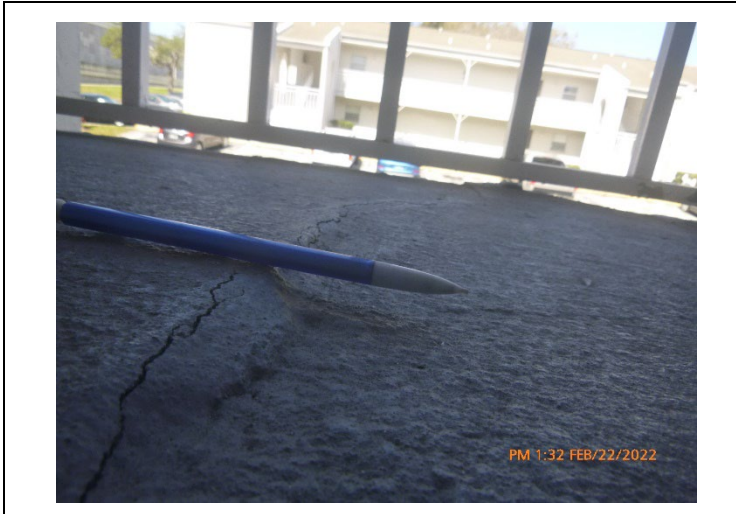
Vertically displaced concrete topping on second floor at Building 5
