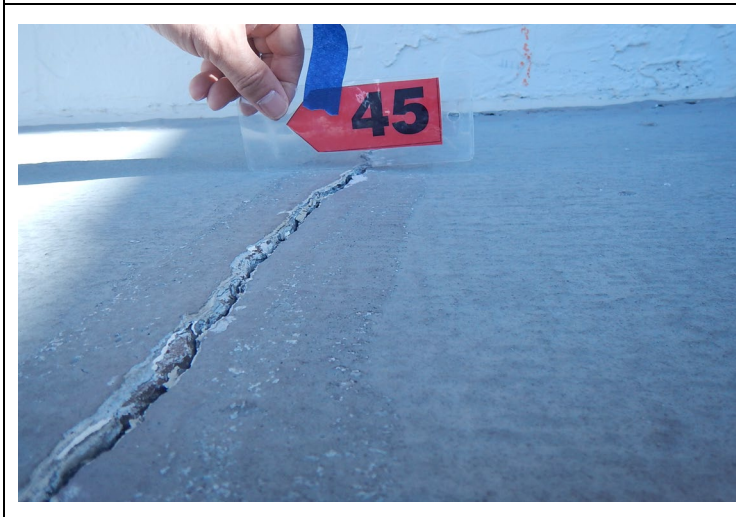
Vertically displaced concrete topping at Building 4
