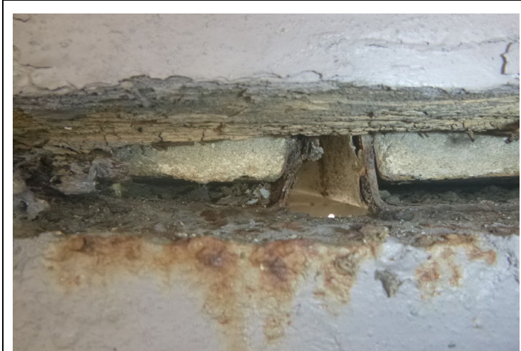
Corrosion and minimal bearing of concrete and metal deck at the stairway landing of Building 11
