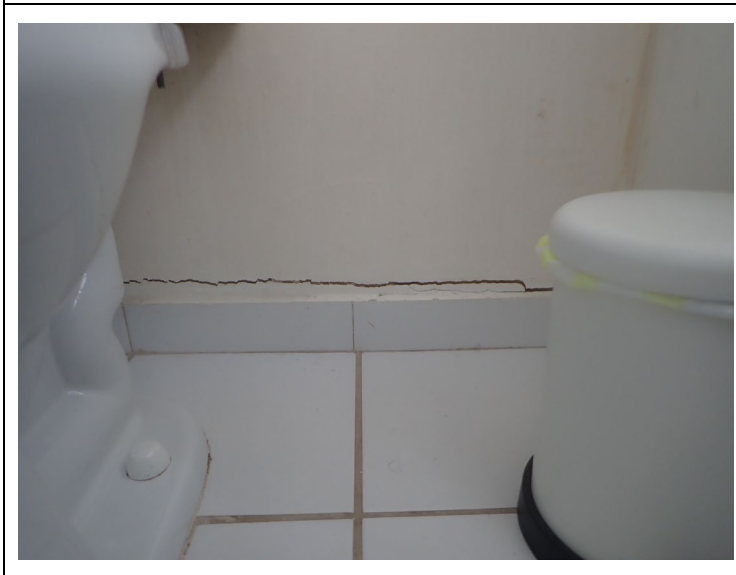
Interior drywall cracking at Building 24 adjacent to cracking at exterior masonry wall
