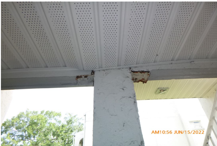
Corroded and distorted metal hangers at Building 19
