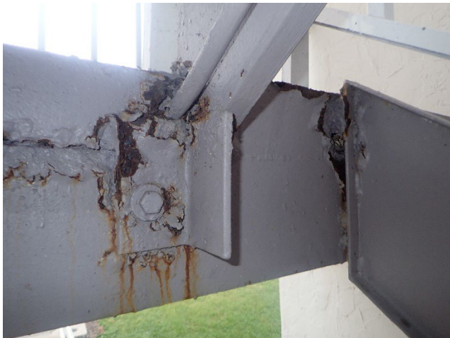
Corroded metal stairs at Building 28
