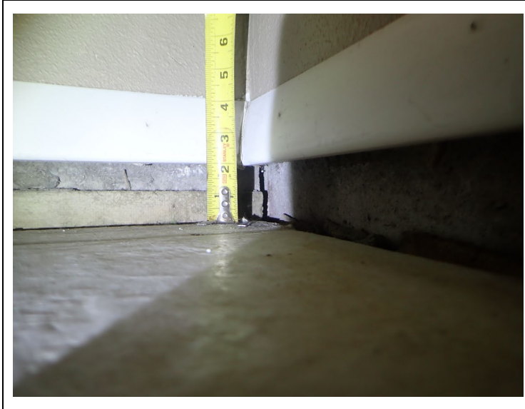
Approximate 2-inch separation of interior concrete floor slab from baseboard at Building 28
