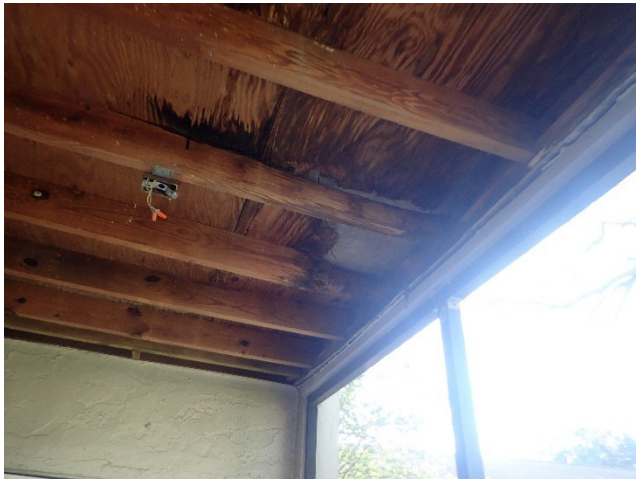
Underlying deteriorated framing at Building 24 after soffit was removed
