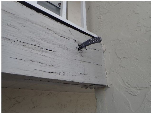
Deteriorated wood beam at Building 12
