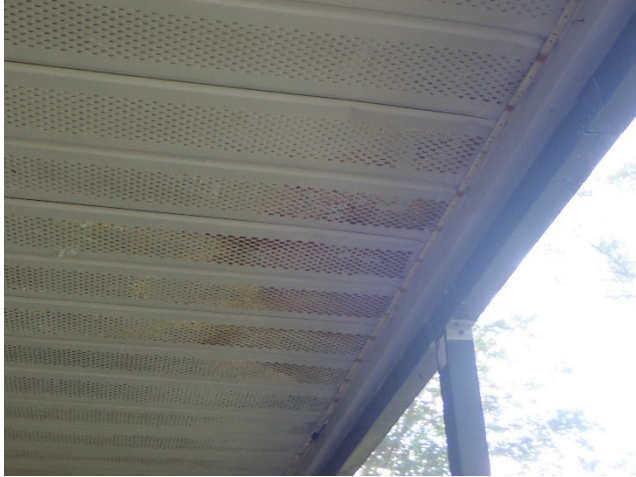
Apparent water intrusion/staining at aluminum soffit at Building 24
