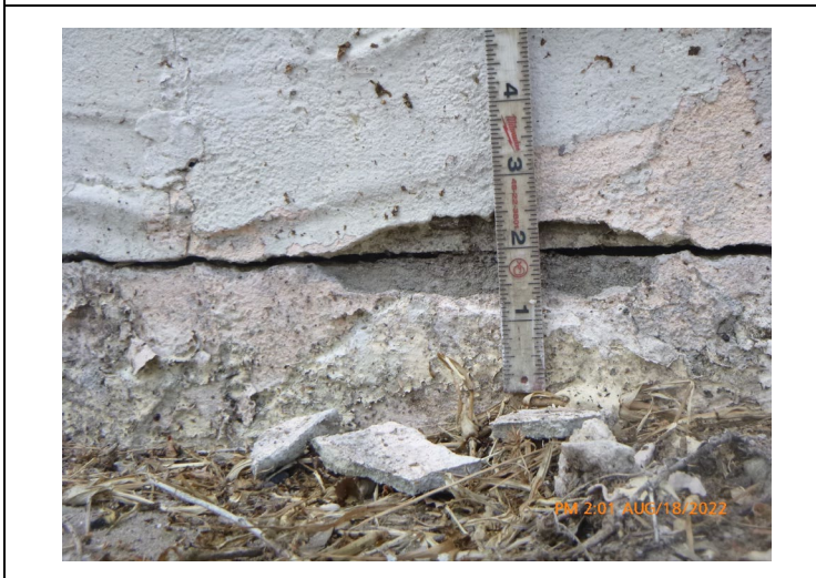
Exterior cracking at masonry wall of Building 24 adjacent to interior drywall cracking
