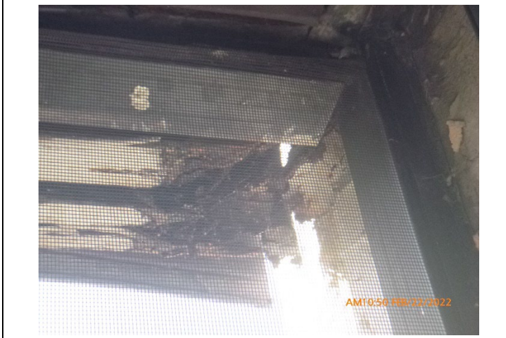
Deteriorated wood beam and deteriorated/corroded metal hanger at Building 5
