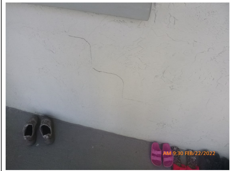
Exterior masonry cracking at Building 5
