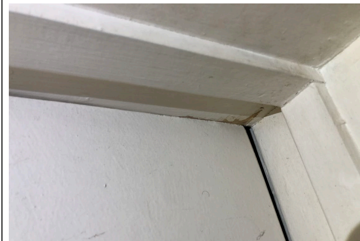
Binding and out-of-square door at Building 4
